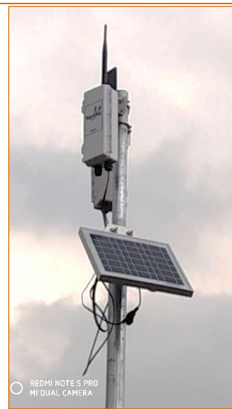
Microclimate monitoring station installed at CAAST-CSAWM, Climate Smart Blocks
